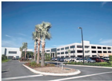
A new building for Gartner is under construction off Chamberlin Parkway in south Fort Myers.
