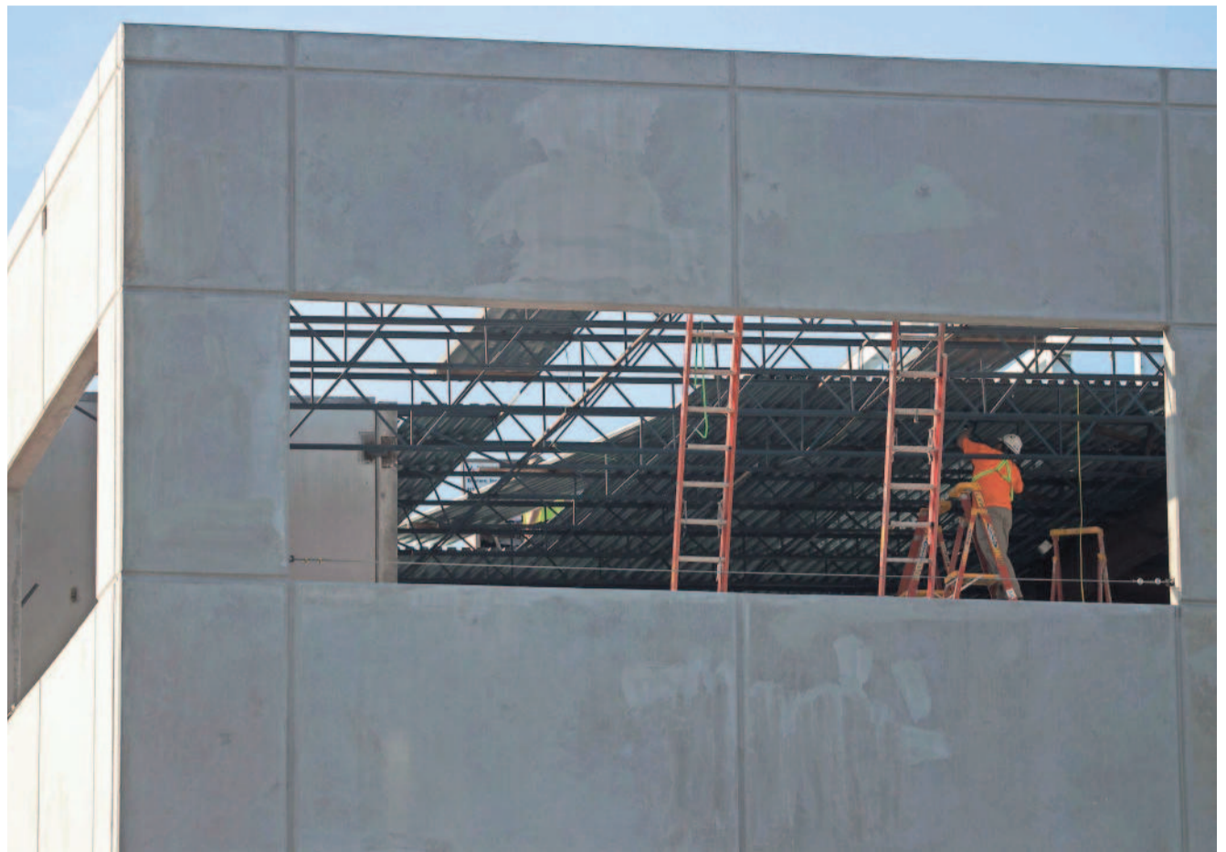
A new building for Gartner is under construction in south Fort Myers and will be a part of a new commerce park near Southwest Florida International Airport. PHOTOS BY AMANDA INSCORE/THE NEWS-PRESS
